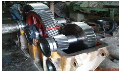
Figure 3. furnace gear reducer
